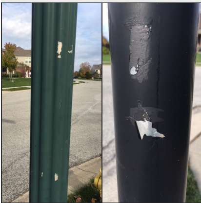
*Examples of recent damage caused by the taping of signs onto light poles.
